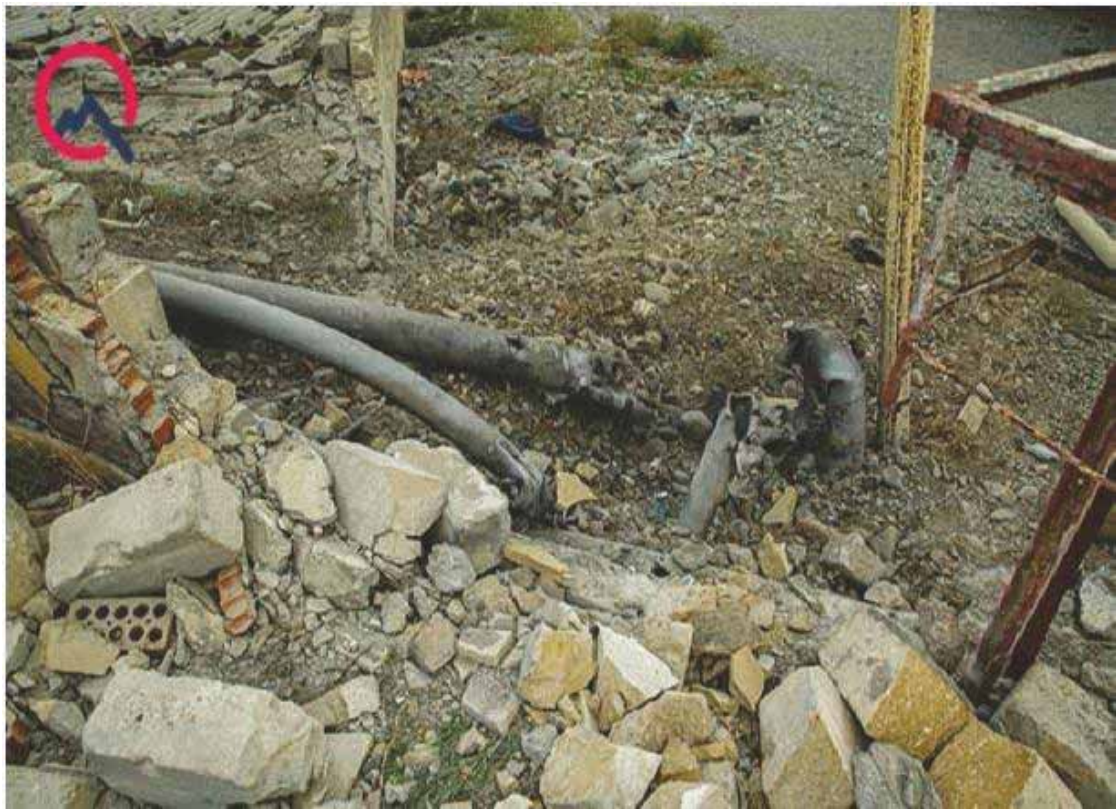
Electricity and energy infrastructure damaged and settlements were cut from electricity
