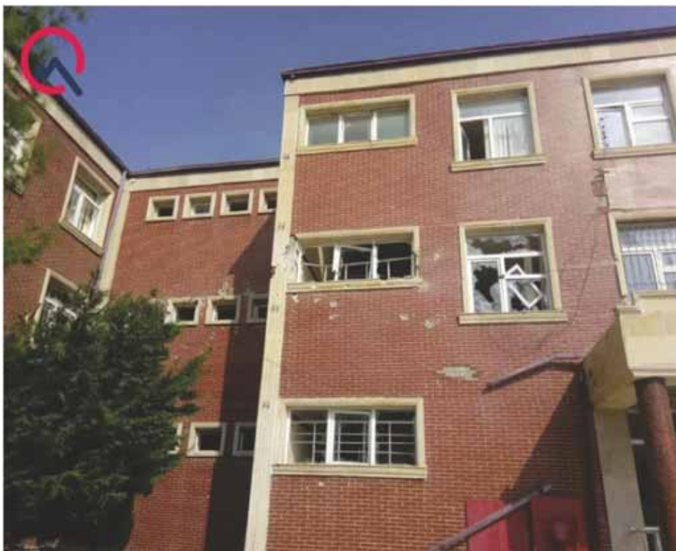
Damaged secondary school No. 1 in Tartar
