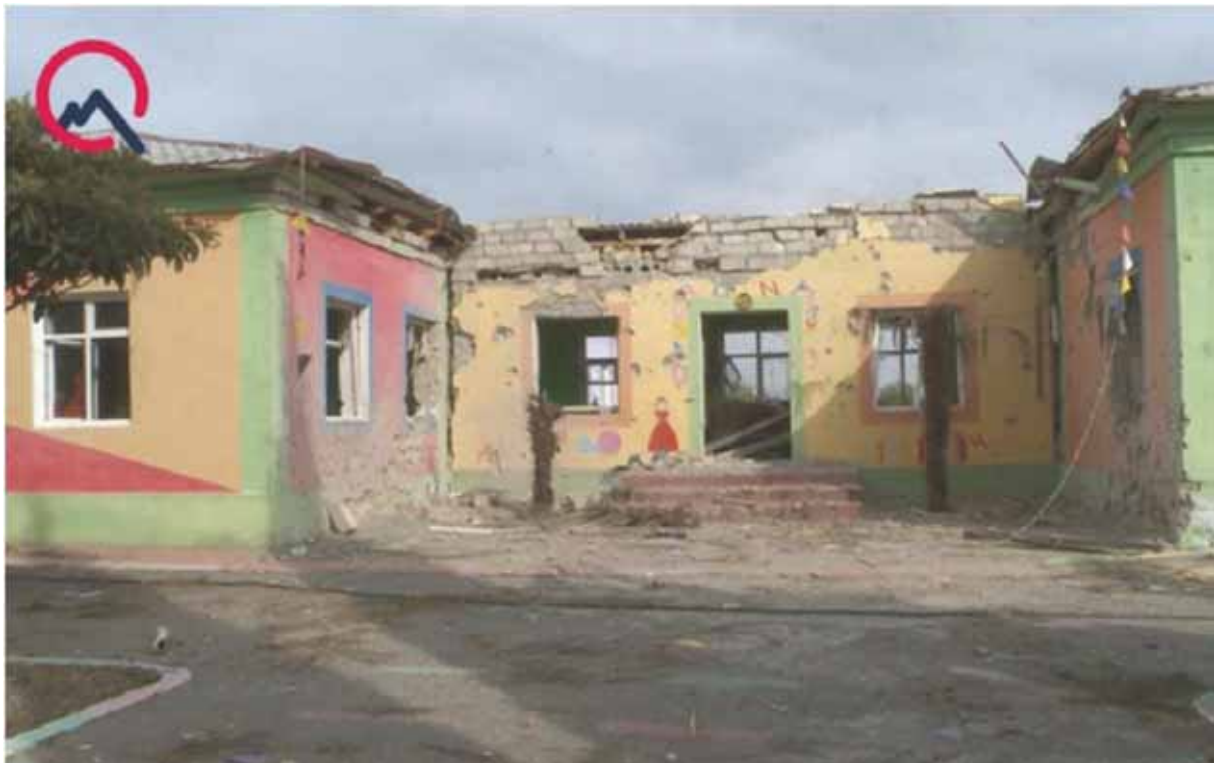
Kindergarten in the Baharli settlement of the Aghdam district damaged as a result of artillery shelling by the armed forces of Armenia on October 26, 2020
