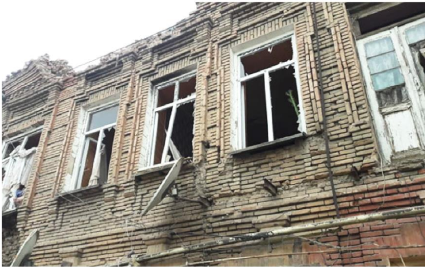
Photo 36: Historical building in the city of Ganja hit by missile
