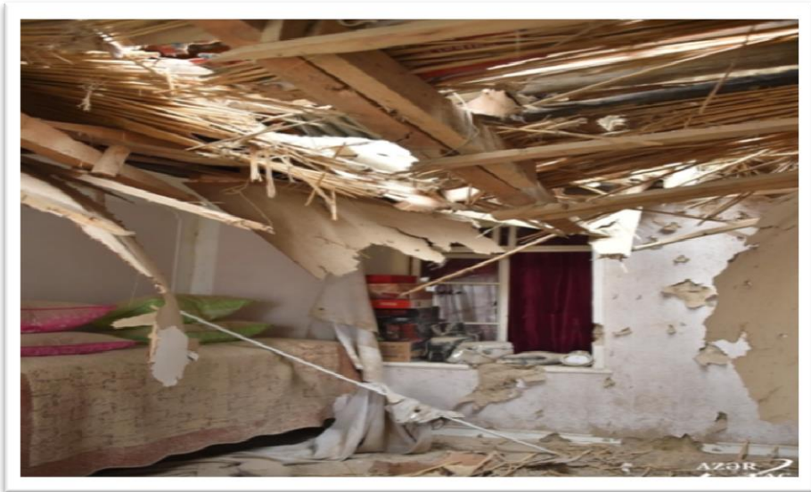
Photo 13: Private property in Goranboy district damaged
