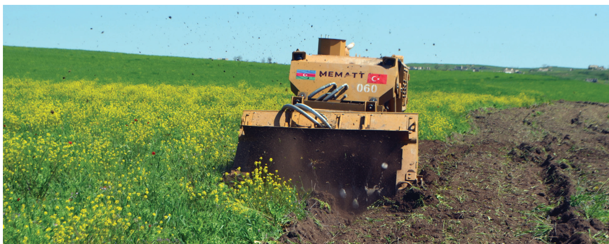
Mine clearance of grassland using MEMATT mine clearance machine, Fizuli district, Azerbaijan
